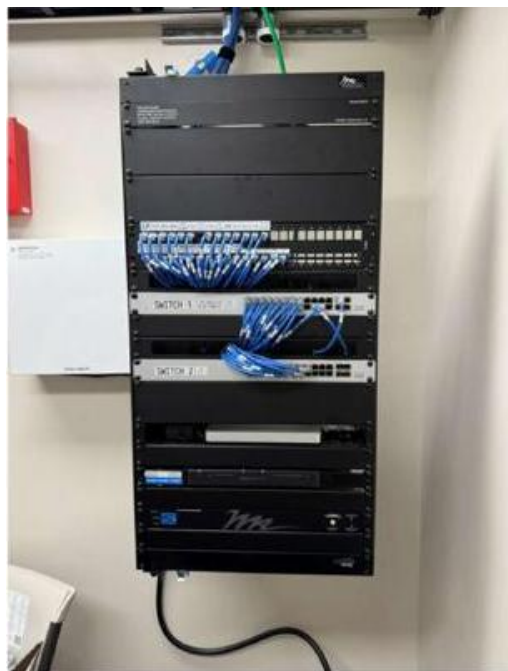
SOW reference photo — wall-mounted enclosed rack with switches and patch panel installed.
