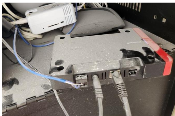
Honeywell LGW1000 installed in an HVAC/BMS closet with network patch connection.
