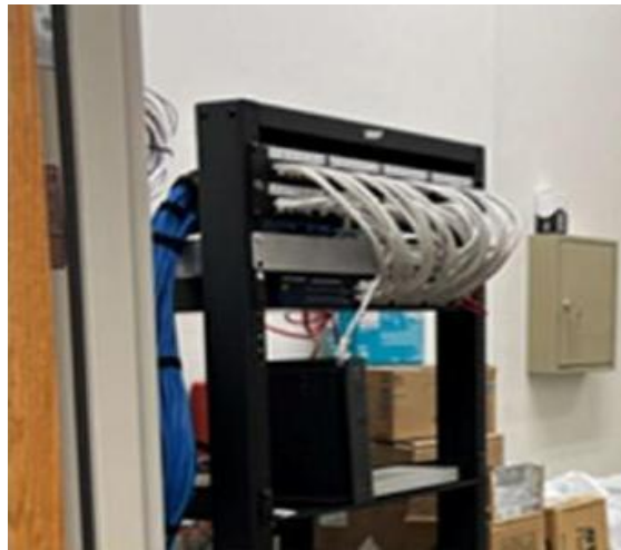
SOW reference photo — open-frame rack installed in an A/V closet with patch cabling dressed to the panel.
