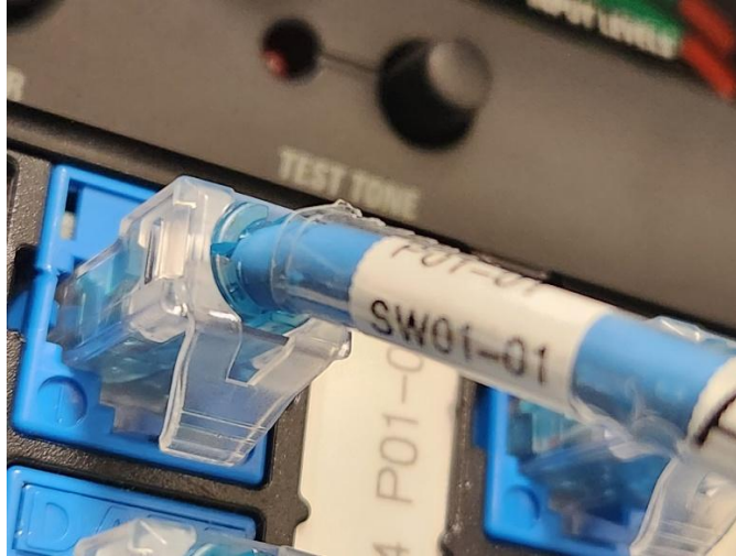
Patch cable labeling example near end – fair end (with device) —labeled by system (AV-1, AV-2/Carrier, HVAC).
