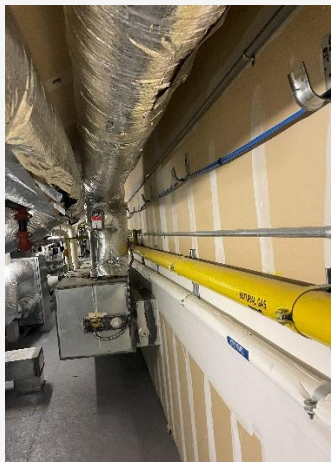
Trunk run supported every 5 ft (minimum) with J-hooks. 1ft distance between other cable runs
